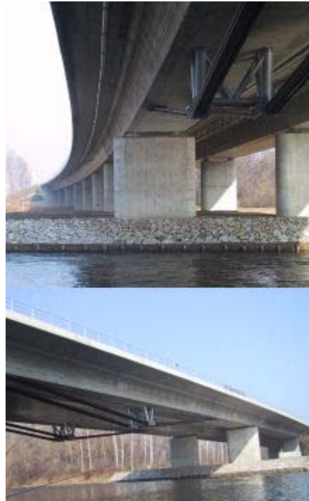
Photos are reprinted by courtesy of Viktor Markelj (designer of the Mura Bridge), Slovenia
